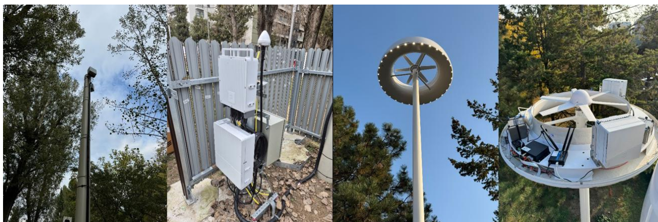
Figure 31. Outdoor 5G radio equipment.
